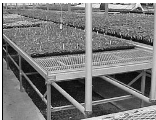
Figure 2. Below bench heating using hot water pipes.
